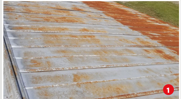
Rusted metal roof
