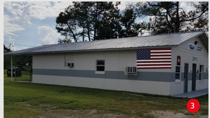
Fully restored roof, brand new look and long term rust protection for up to 90% less cost than a roof replacement
